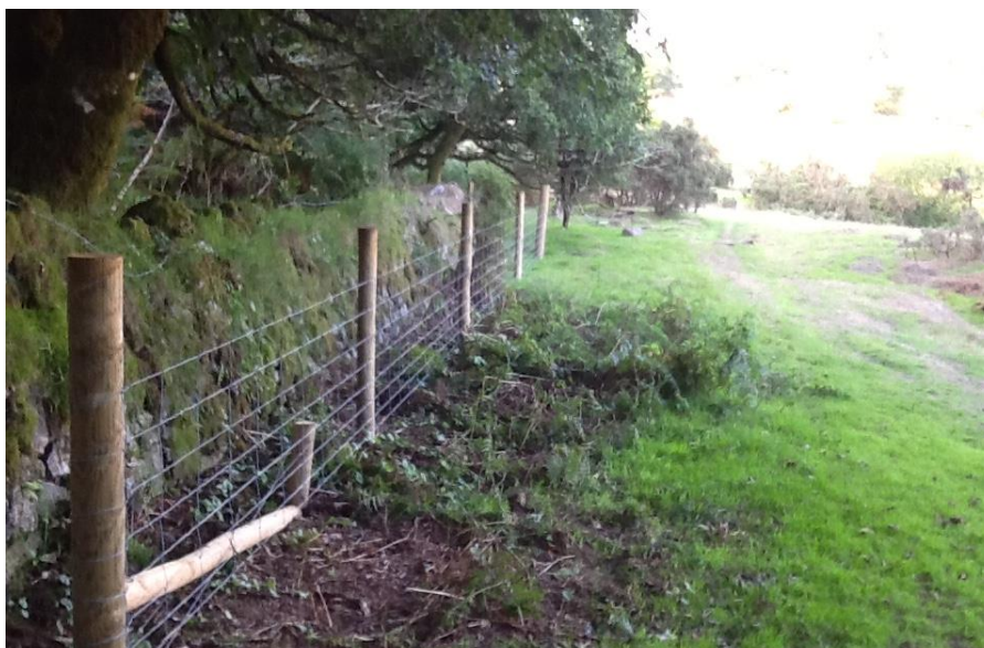
New fencing inside of SAM from south looking north Photo: Iain Rowe
